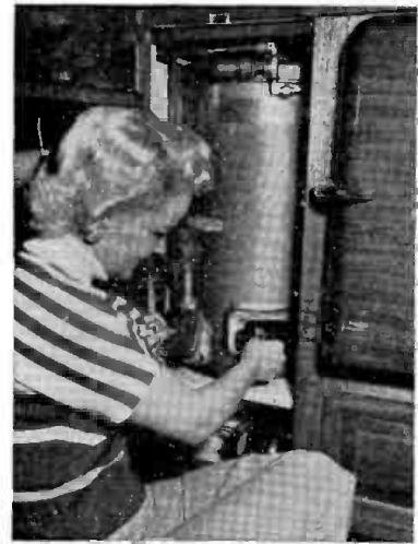
Sea-Going Water Heater. This space-saving 7 gallon storage water heater operates on butane gas to provide hot water up to 180° in a 30-foot Tahiti ketch. Running hot water, like many other "comforts of home," is usually ruled out on a small ship because of space restrictions. But this midget heater, made of USS Steel Sheets, is just the ticket for small craft.
