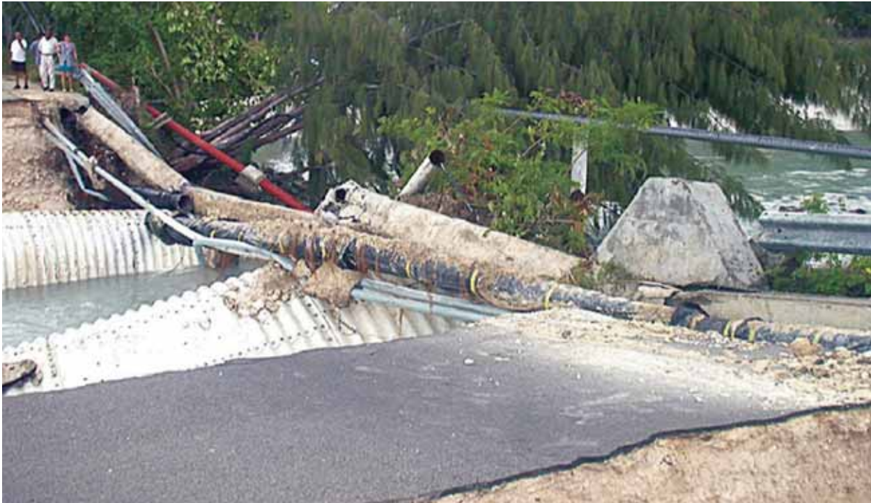
Victoria suffered the most extensive damage in the Seychelles, particularly to infrastructure such as bridges, roads, port facilities and sewage systems.
