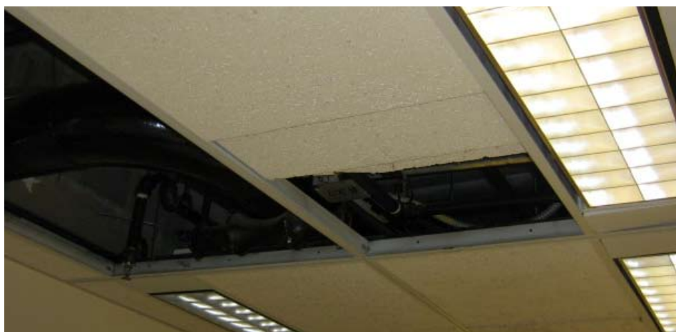
Figure 1: Missing and damaged ceiling tiles
