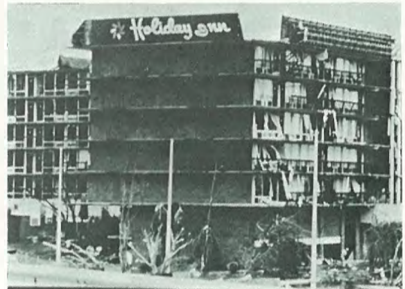
Above: A view of some of the wind damage to NHC's communications equipment atop the IRE Financial Building. The radar dome of the WSR-57 weather radar was blown off the highest structure seen at the center right of the photograph. (Photo courtesy: Roger Edwards)
