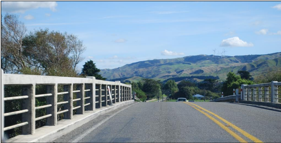
Figure 62: Many railway overbridges have inadequate shoulder width and may require clip-on bridges on each side for cycling safety (photo: Jonathan Kennett)
