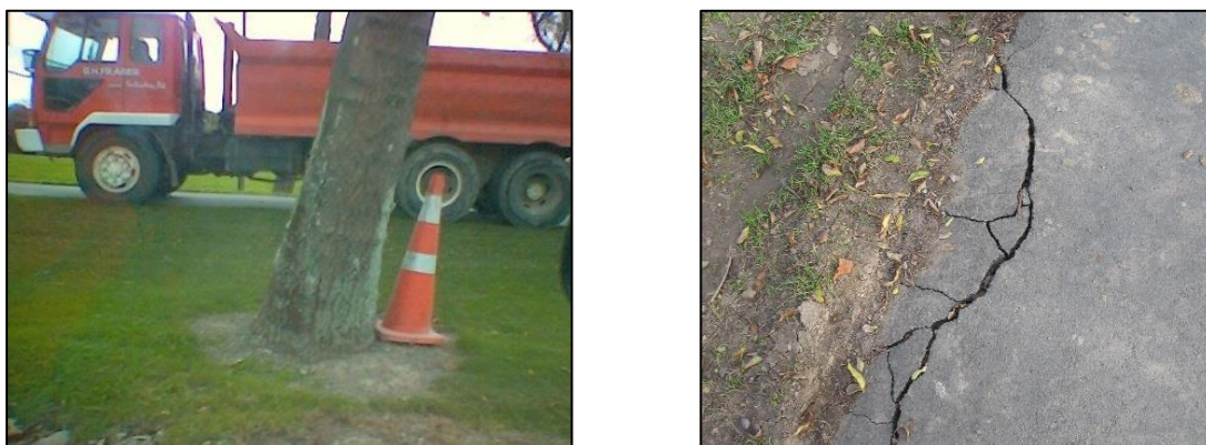
Figure 30: Heavy truck causing edge break on new pathway during construction
