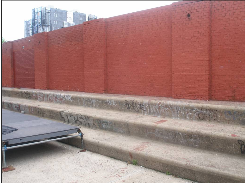
McCarren Play Center filter house: bleacher area, looking northeast. Photo: Kathryn Horak, 2007
