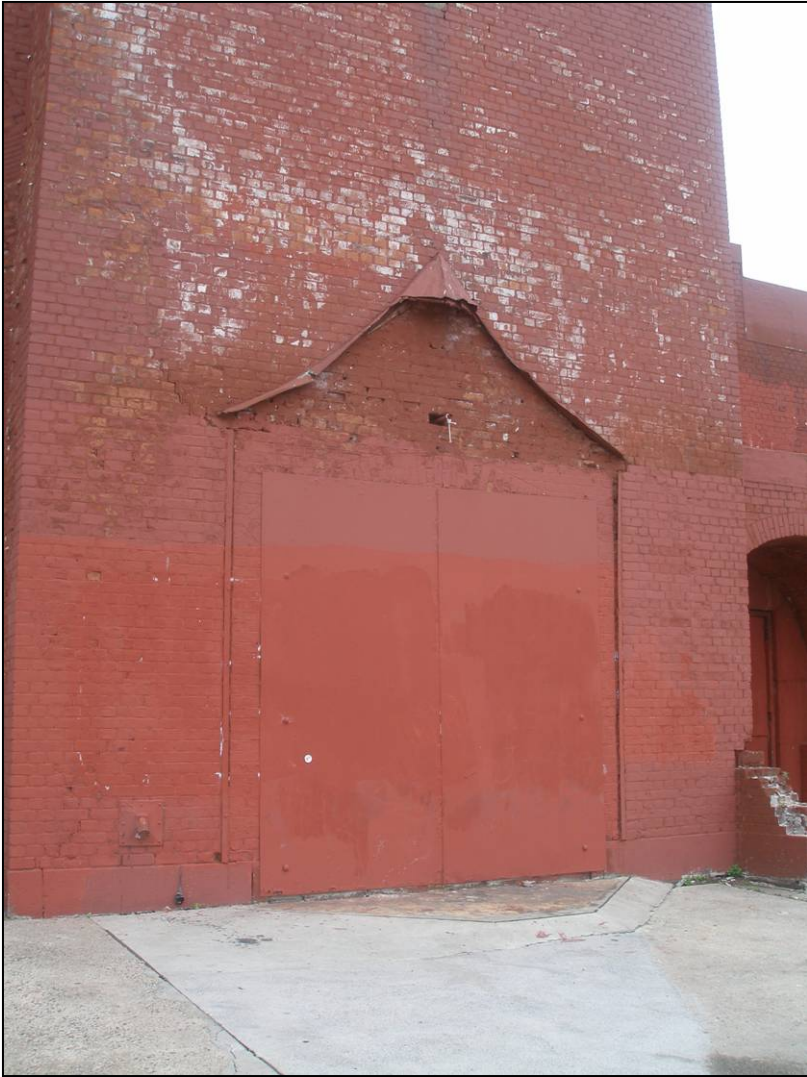
McCarren Play Center bath house: East façade, remnants of glazed bay, north tower, looking west. Photo: Kathryn Horak, 2007
