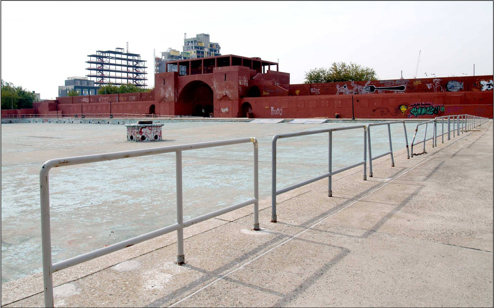
McCarren Play Center: swimming pool and bath house, east façade, looking southwest. Photo: Zerina Philip, NYC Parks Dept., 2006
