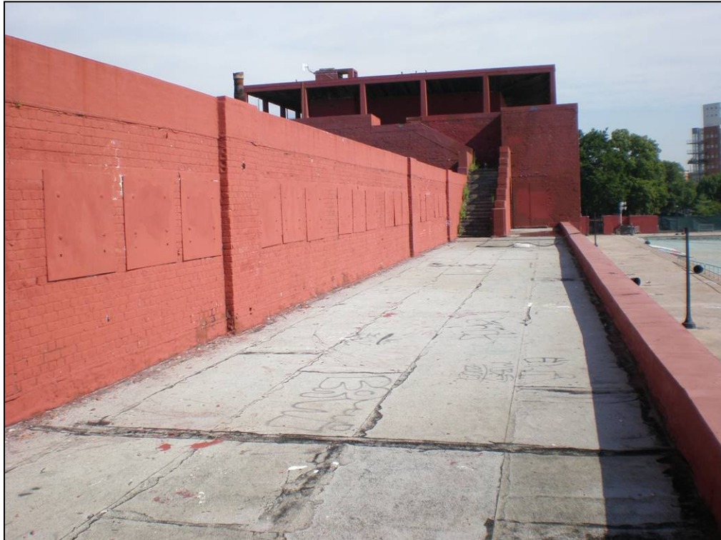
McCarren Play Center bath house: viewing platform, south wing, looking north. Photo: Kathryn Horak, 2007
