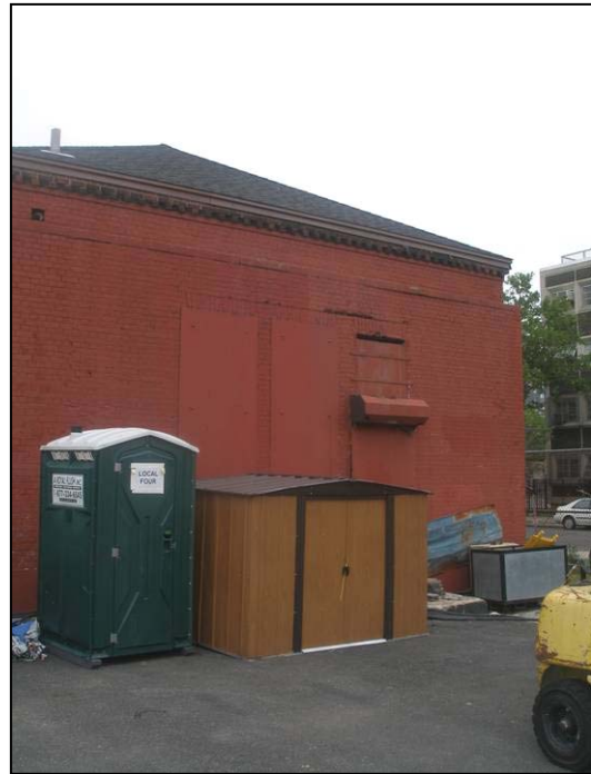
McCarren Play Center filter house: south façade of southern filter house building, looking northeast.
