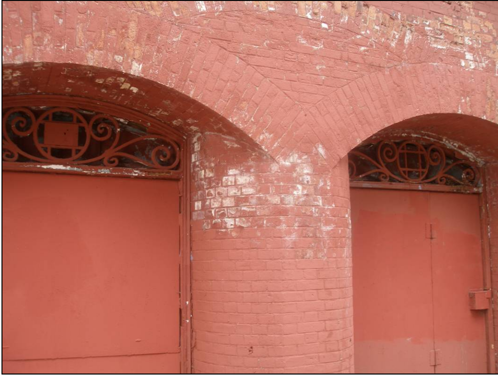
McCarren Play Center bath house: pavilion interior, entrances to north wing. Photo: Kathryn Horak, 2007
