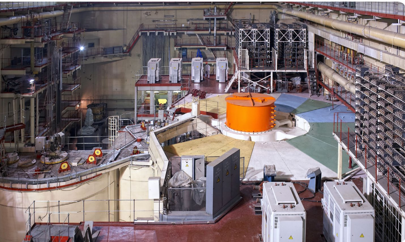
BN-600 reactor hall
