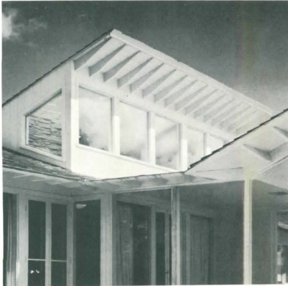
Fig. 17 HOOD OVER WINDOW designed to admit winter sun, exclude summer sun, and equalize the light inside the room
