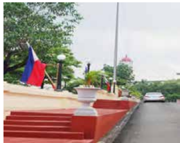
The restoration and repair works at the podium and west driveway have been partially completed in 2010. Works involved were repair of electrical system, repainting of the concrete surfaces.
