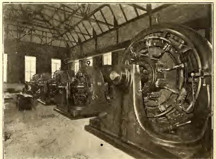
INTERIOR OF CONEY ISLAND SUB-STATION
