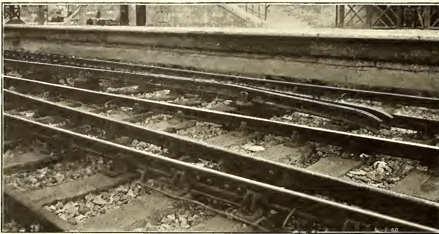
SECTION OF THIRD RAIL AT CHAMPS DE-MARS STATION, SHOWING DOUBLE INCLINE, ALSO METHOD OF RETURN-CIRCUIT BONDING
