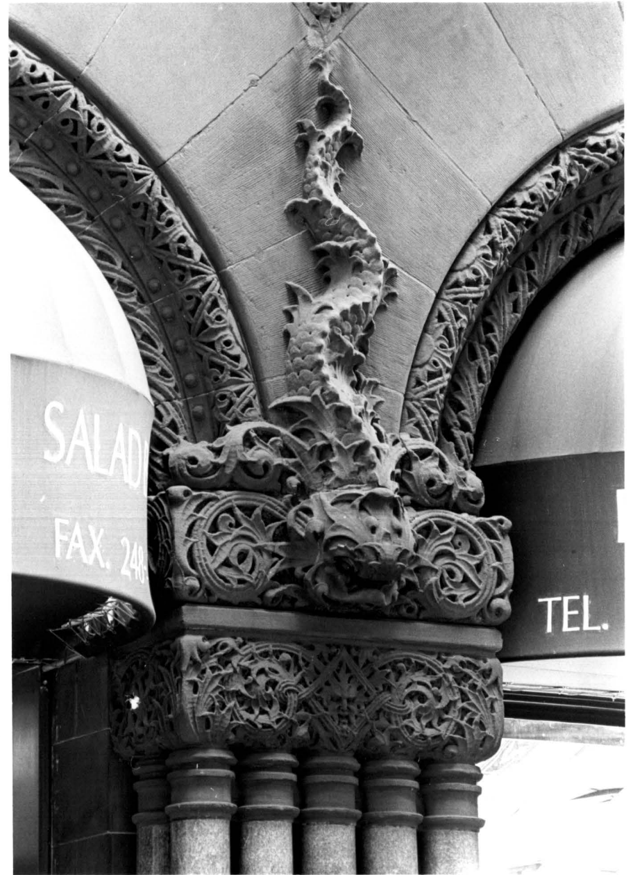
56-58 Pine Street Building, ground story detail, Pine Street facade Photos: Carl Forster
