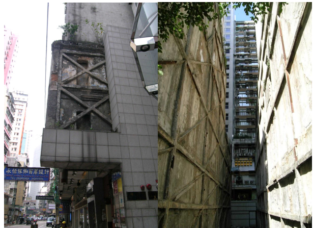
Fig. 4 Party wall in between two previous Tong Lau (first photo) and skeleton of party wall remaining on side walls of buildings (second photo), Queen's Road East, Wan Chai, Hong Kong.
