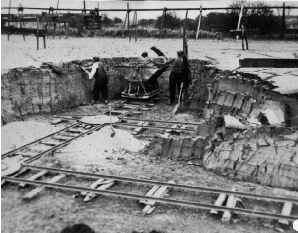
Excavating a washback in one of the larger Eastwood brickfields in the 1900s. The slurry launders can be seen in the background.
