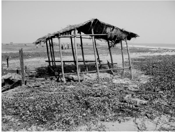
Fig. 6. Damaged hut in Kapyet Thuang Village.
