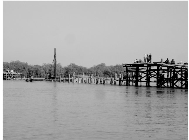
Fig. 7. Destruction of wooden bridge to Plautonton Island.
