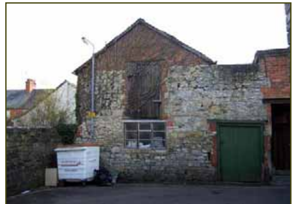
Figure 28 Outbuildings, The Causeway - in need of a sympathetic reuse
