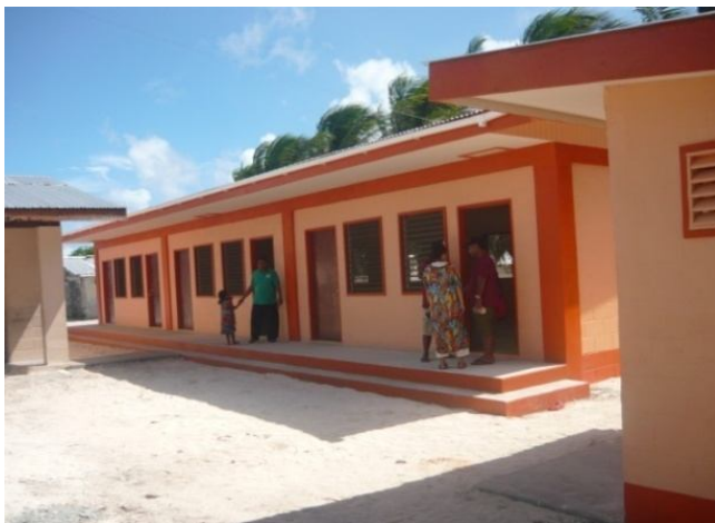
MOE Maintenance Crew working on three new classrooms at Ulien Elementary School (Arno). Funded by Japanese Grassroots.
