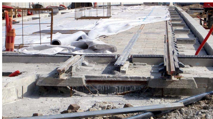
Figure 9: Typical Embedded Track with embedded third rail during construction in Bordeaux, France
