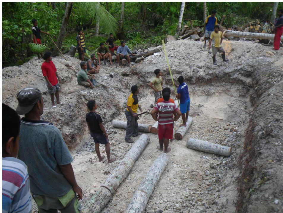
Figure 18: Coconut palm tree trunks/logs were laid, in special arrangement, at the bottom of the lase hole. Older experienced men were directing the younger ones how to do the lay-out
