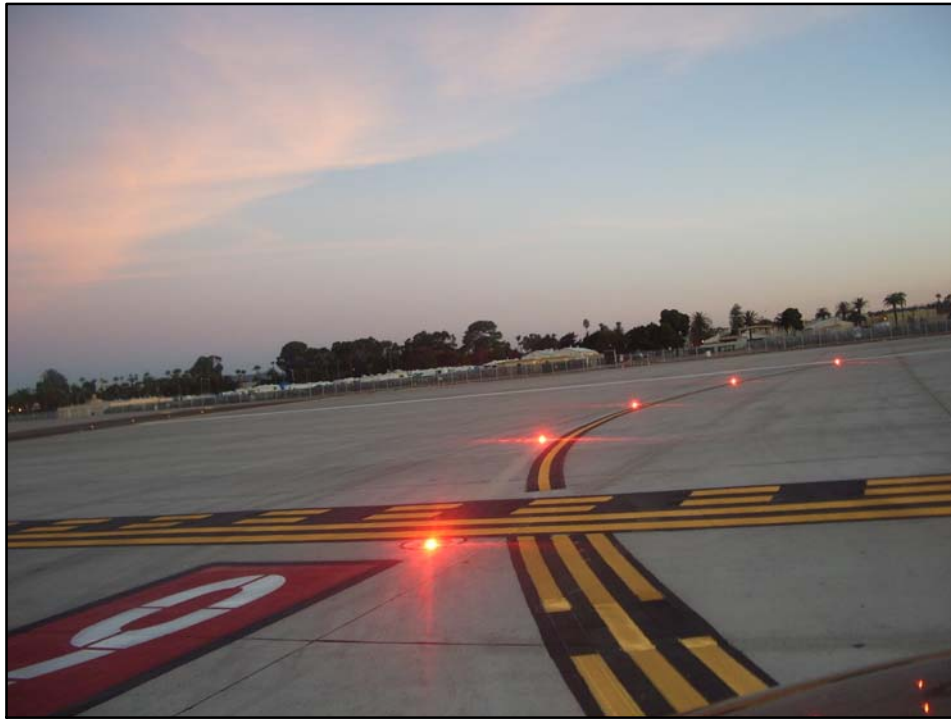
FIG 2-1-12 Runway Entrance Lights
