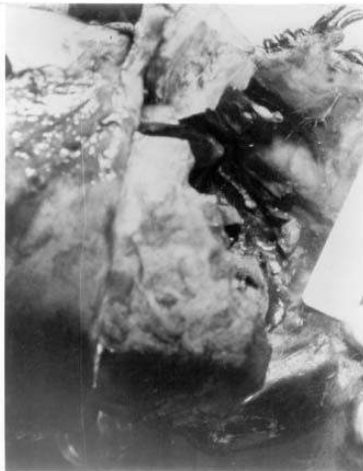
Above - Detail of Large Defect
