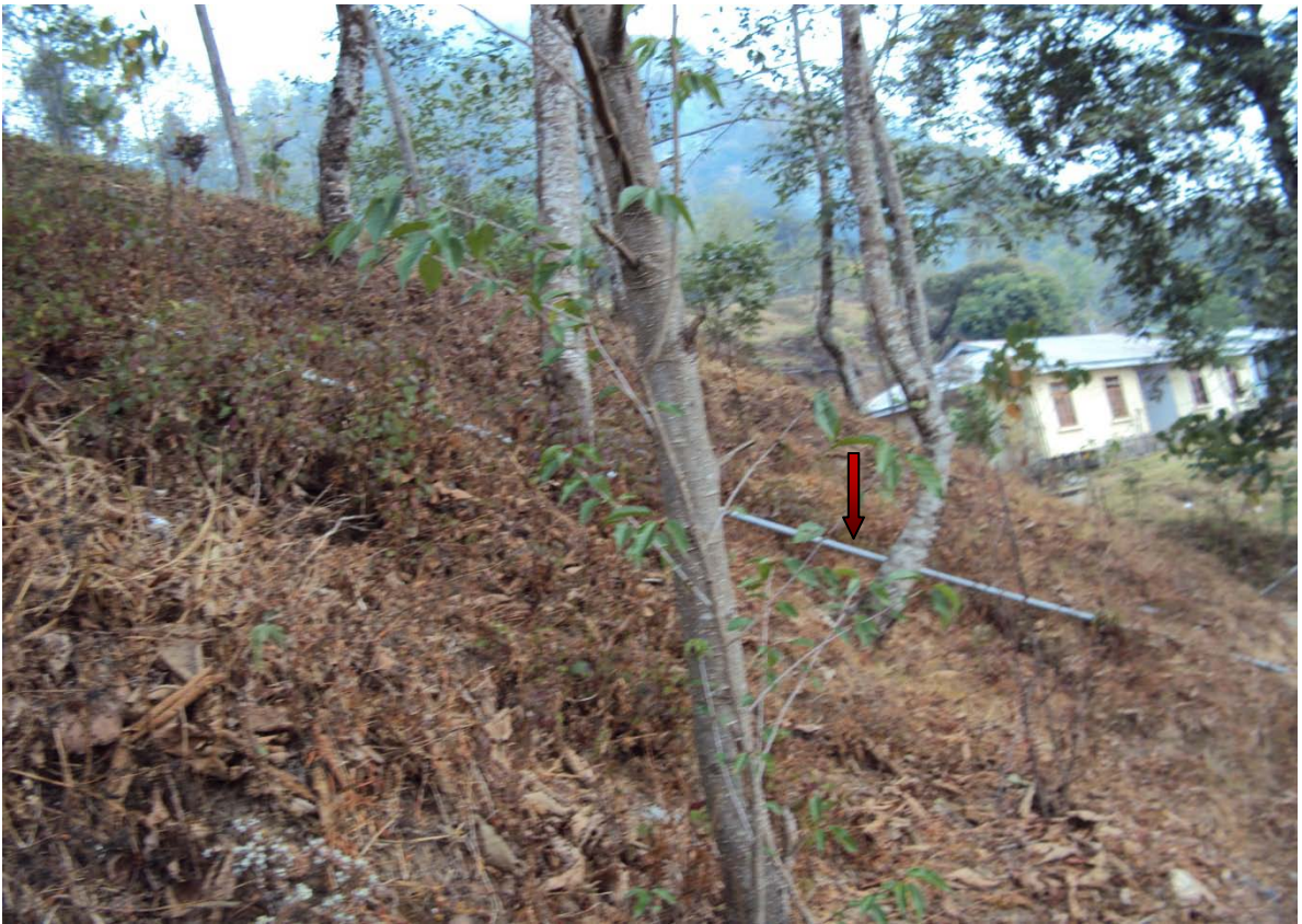
Distribution pipe line from the Reservoir
