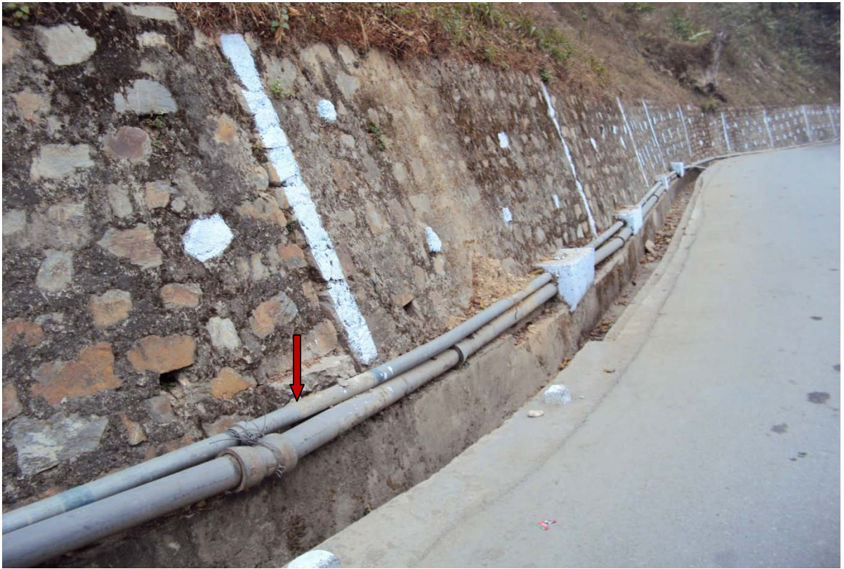
Distribution Pipe Line to Namchi Town
