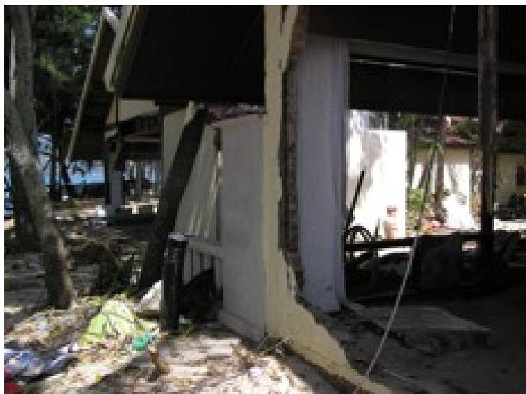
Photo 4.11 The broken wall of a house built of brick at Patong beach
