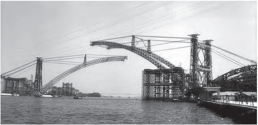
Figure 17.20 Construction of Yajisha Bridge (Photo: Engineer Leo K.K. Leung, Executive Director of Hopewell Highway Infrastructure Ltd (Hong Kong Stock Code: 737))
