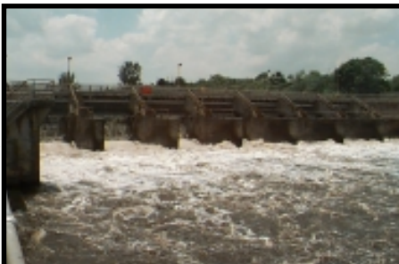
S-80 Structure at the east end of C-44, during a high-flow discharge in the May 2000 drawdown of Lake Okeechobee.
