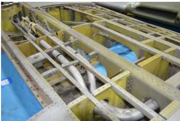
N13Y Radiator/Oil Cooling Tubing in Wings
