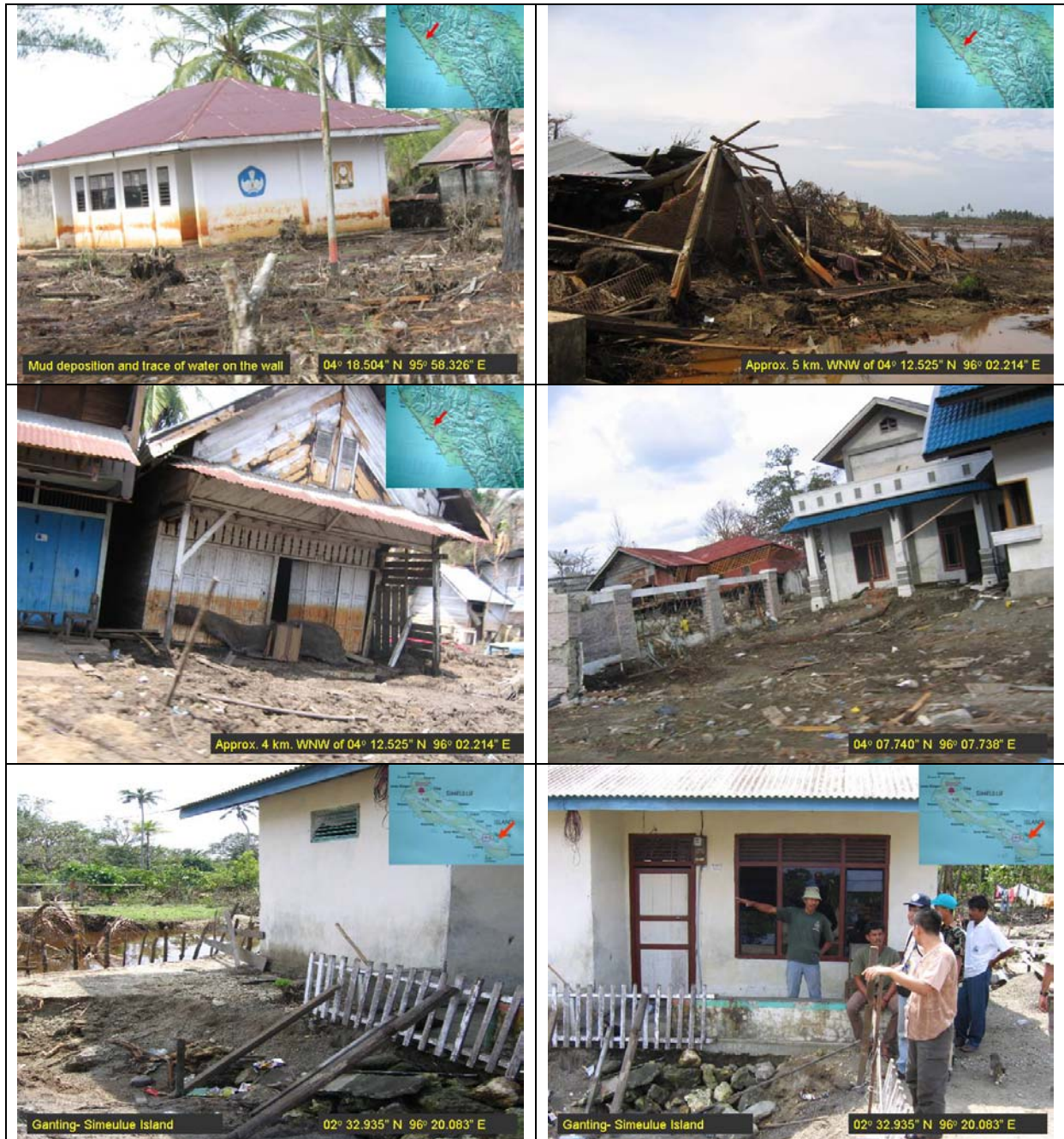
Figure 8: The typical damages and damage levels of tsunami on concrete structures.
