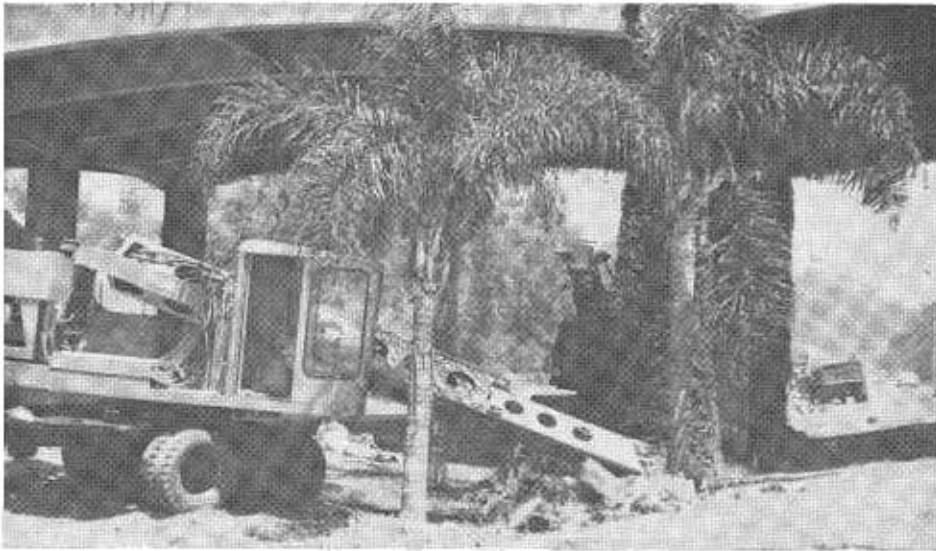
The start of excavating operations to salvage a palm tree from the median strip of the Cabrillo Freeway.
