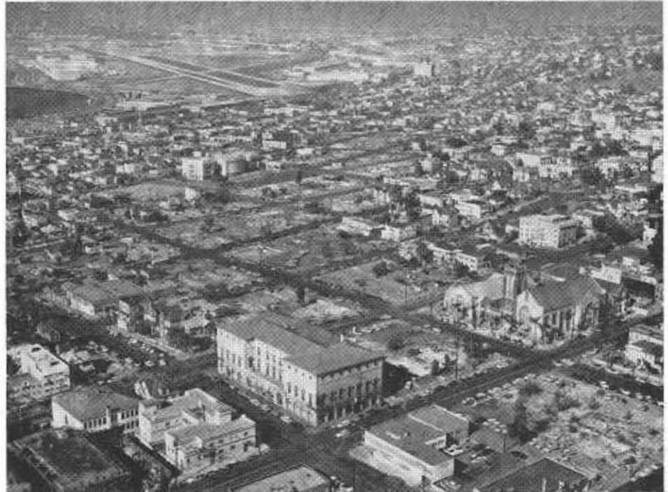
Cleared areas for freeway construction in San Diego can be seen in the above photo beginning lower right and ending upper middle.
