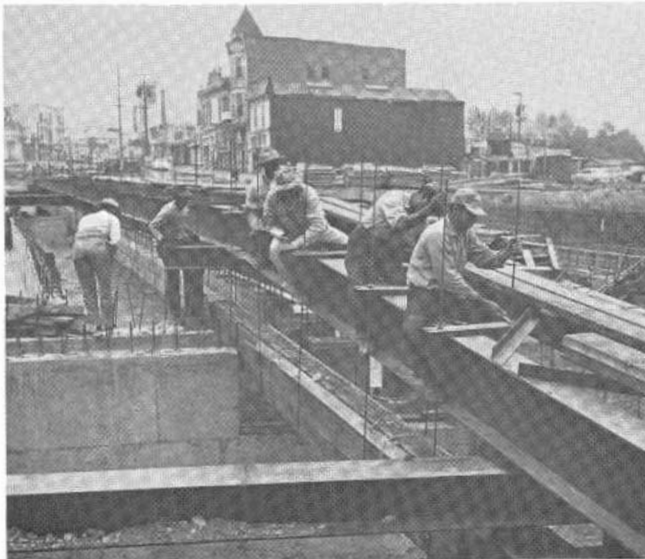
Workers prepare to release the steel straps and lower the ducts into their final position inside the concrete girder.
