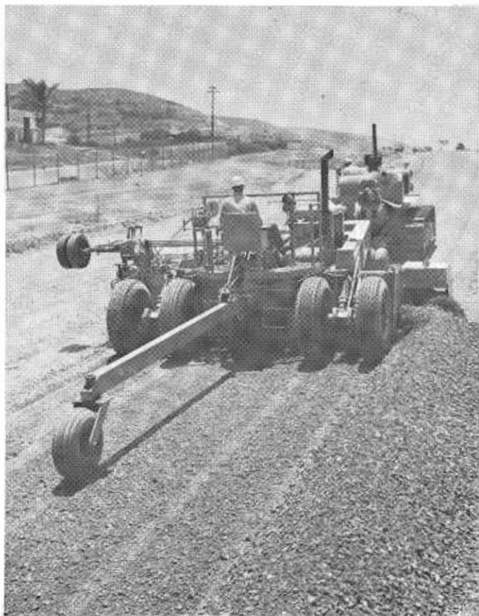
Automatic road building machine cuts subgrade on untreated base. Stakes carrying the grade wire are on the left in front of the machine.
