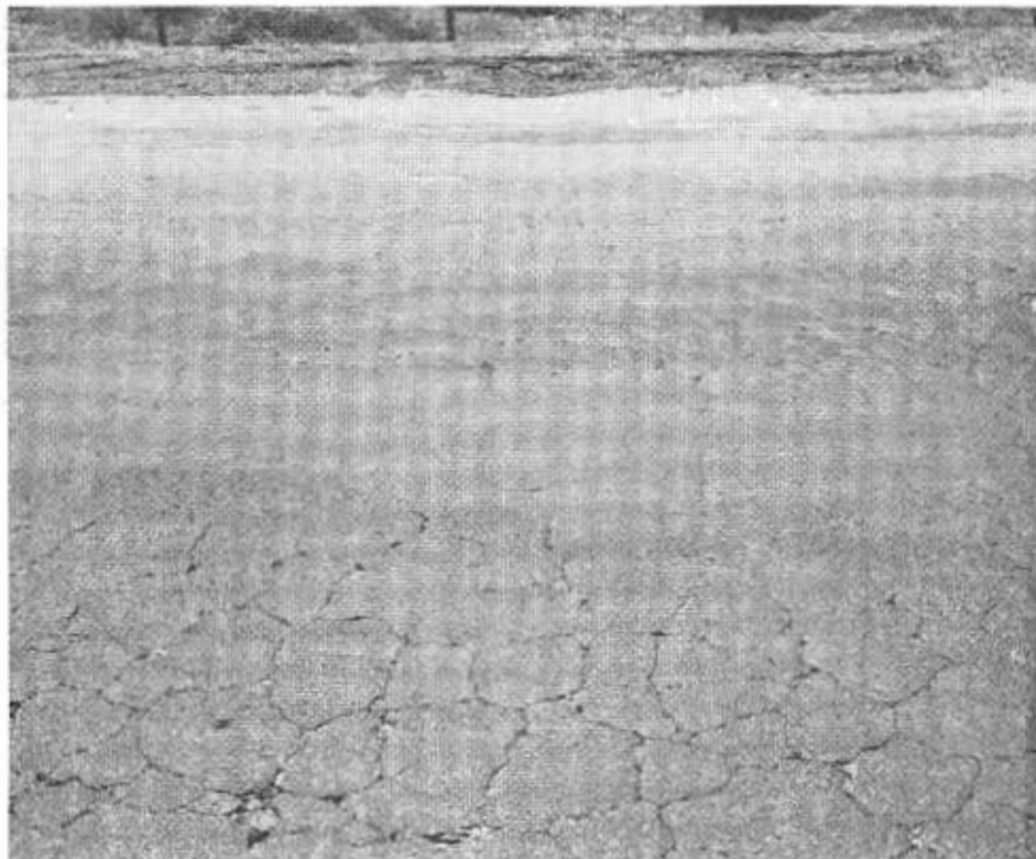
Figure 1. Fatigue cracks, generally known as "alligator" cracks.
