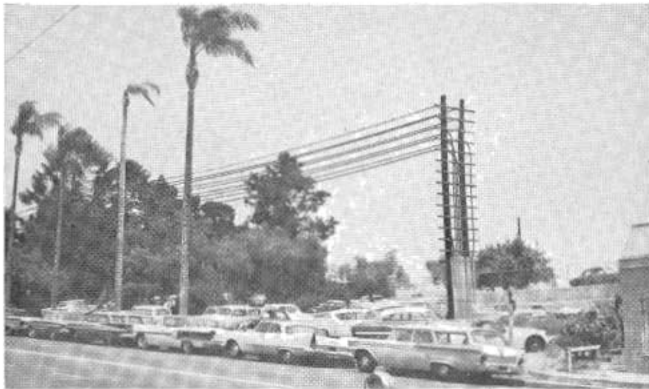
Underground telephone lines were temporarily detoured by leading them out of the ground and suspending them between poles as in the above photo taken at Sixth Avenue.
