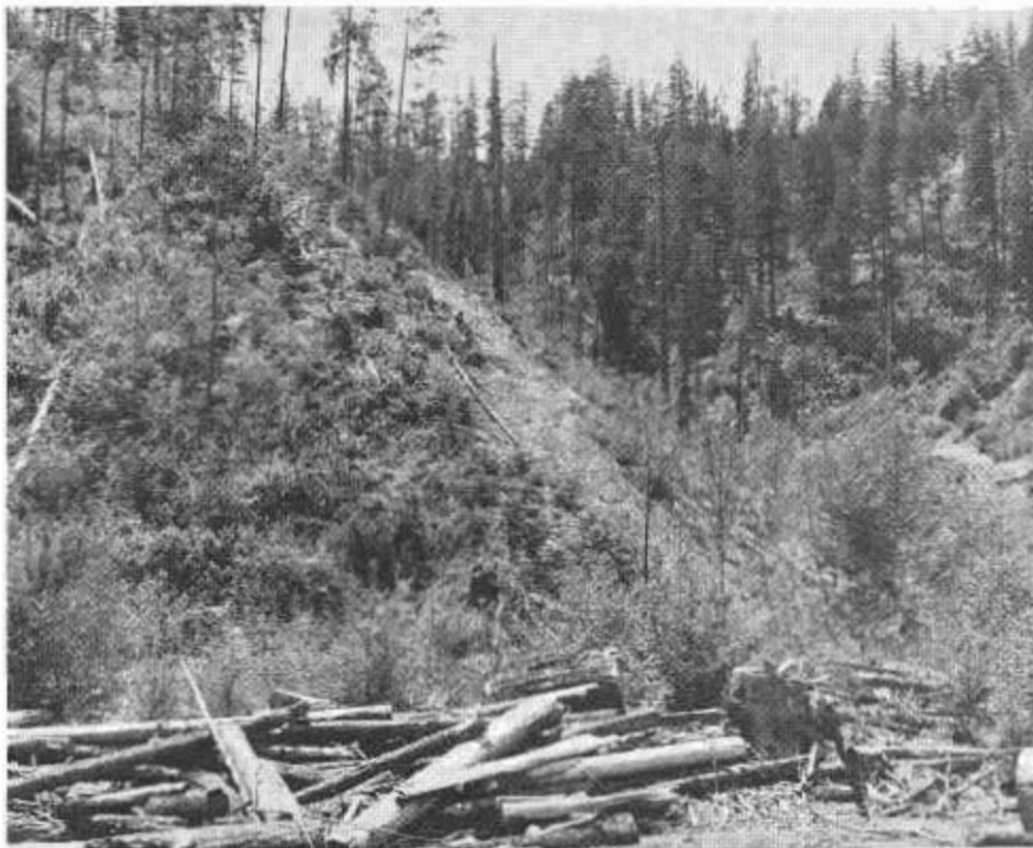
The new road will ascend from Broken Kettle Creek (foreground) up the side canyon and enter the tunnel approximately 150 feet above the creek bed and about 900 feet to the south. The fill across the creek valley will be about 110 feet high.
