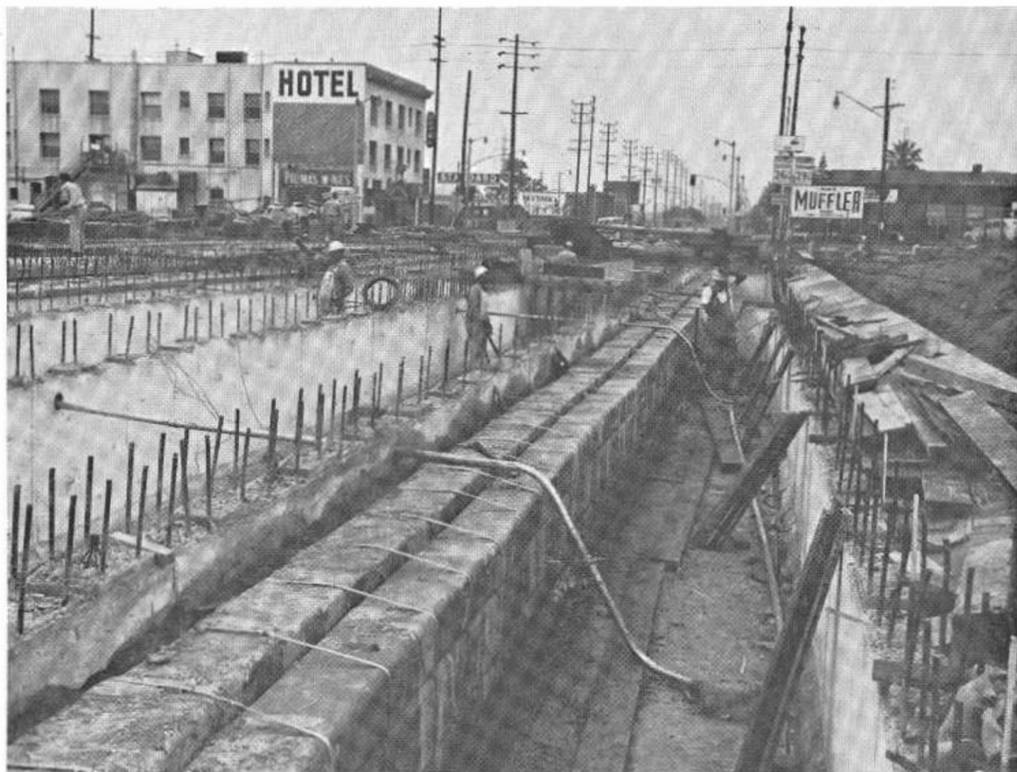
The telephone ducts shown in their permanent position inside the concrete box girder.
