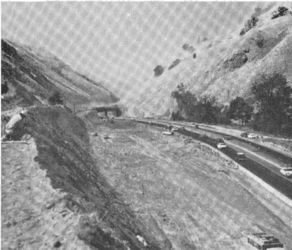
A temporary bridge was constructed over the highway for earth hauling purposes. Part of the old parabolic concrete divider can still be seen to the left of the road on the lower right part of the photo.
