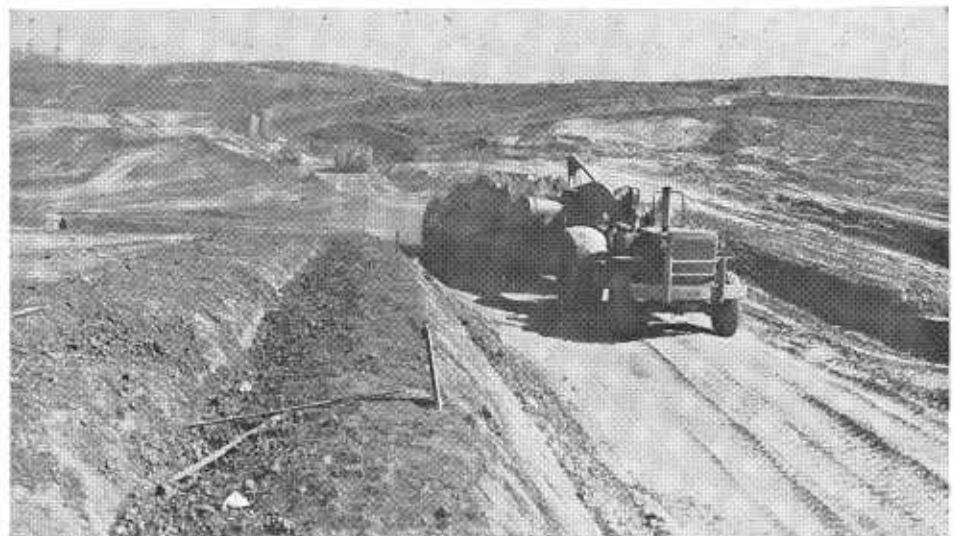
The Nicolas Avenue extension (between the Cities of Fullerton and LaHabra) is being built on a new alignment, financed through the Arterial Highway Financing Plan.
