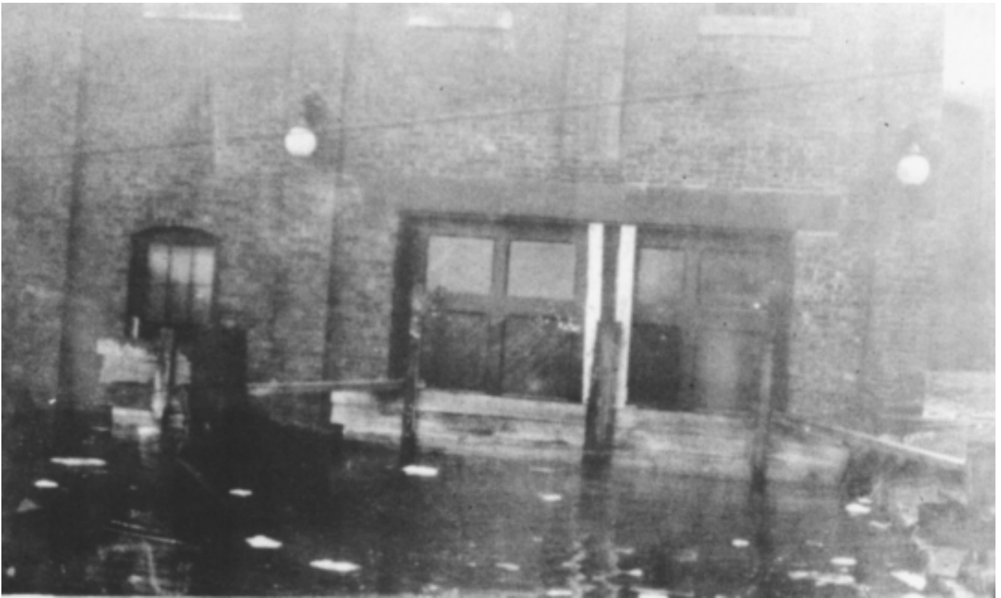
MARCH 1936 - Heavy rains and melting snows cause flooding at Veazie Hydro Station - Upstream end of Veazie Station, showing main entrance with board barricade to keep water out of the station.
