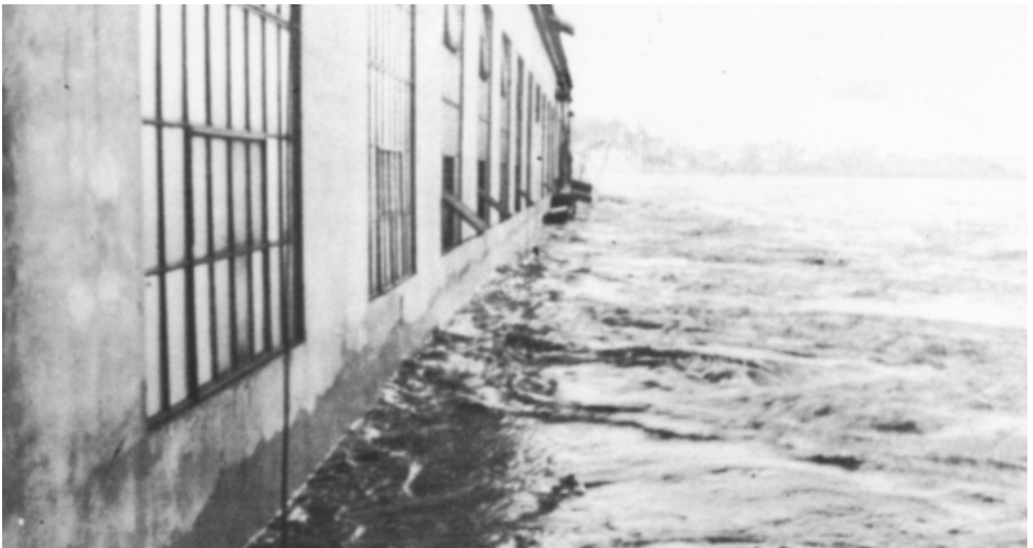
High water in Forebay at Veazie Station, showing outside wall of generator room. Platform which runs entire length of station used for track for rack rake under water.
