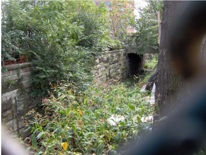
Parcel B6804, looking south from the east side of Third Avenue towards East 156 th Street
