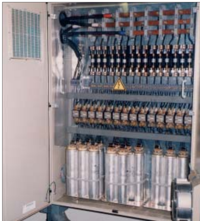
Figure 1: Control and Switching Cabinet for Induction Generator Wind Turbine, Showing Capacitors Mounted in Lower Region to Minimize Heating
