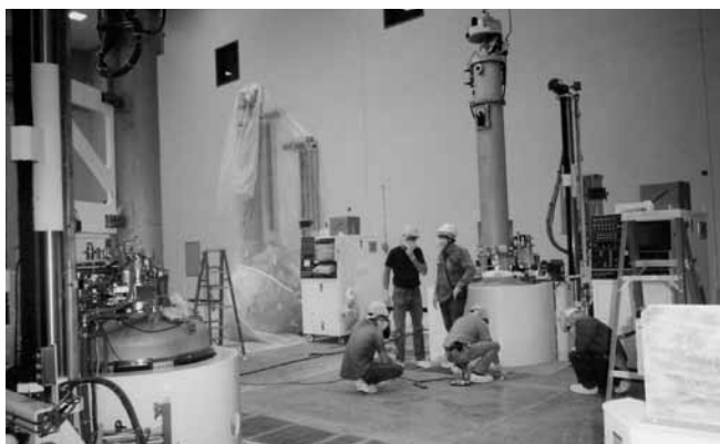
Crystal puller, first tool installed at MEMC Southwest, November 1996.
