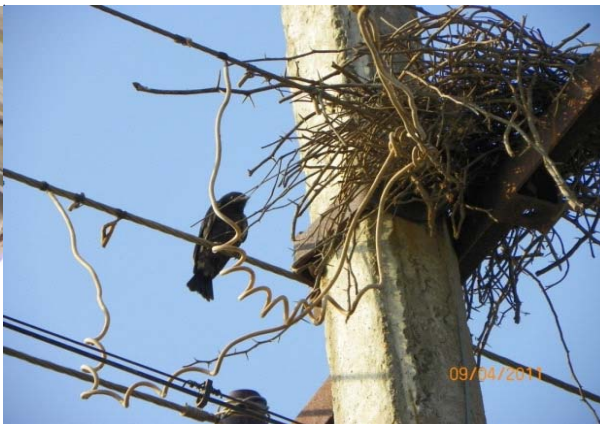
FIG 5 Nesting of Black Drongo on a electric pole
