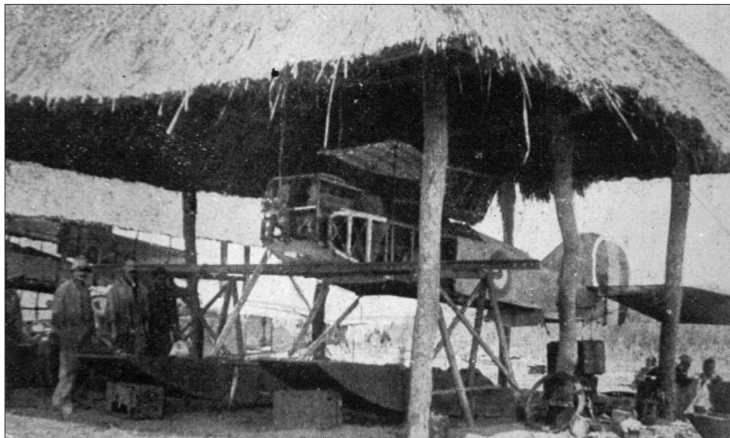
This scene may show the repair of the second Short to be assembled, following its crash and recovery from the shallow waters of the Tongwe lagoon. Another machine stands with wings folded under its adjacent shelter, necessary to protect dope and fabric from the effects of strong sunlight. :Royal Military Museum, Brussels
