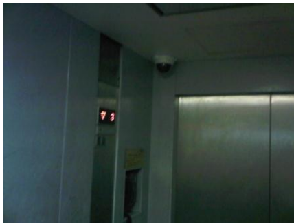
Security camera in oversize baggage elevator
