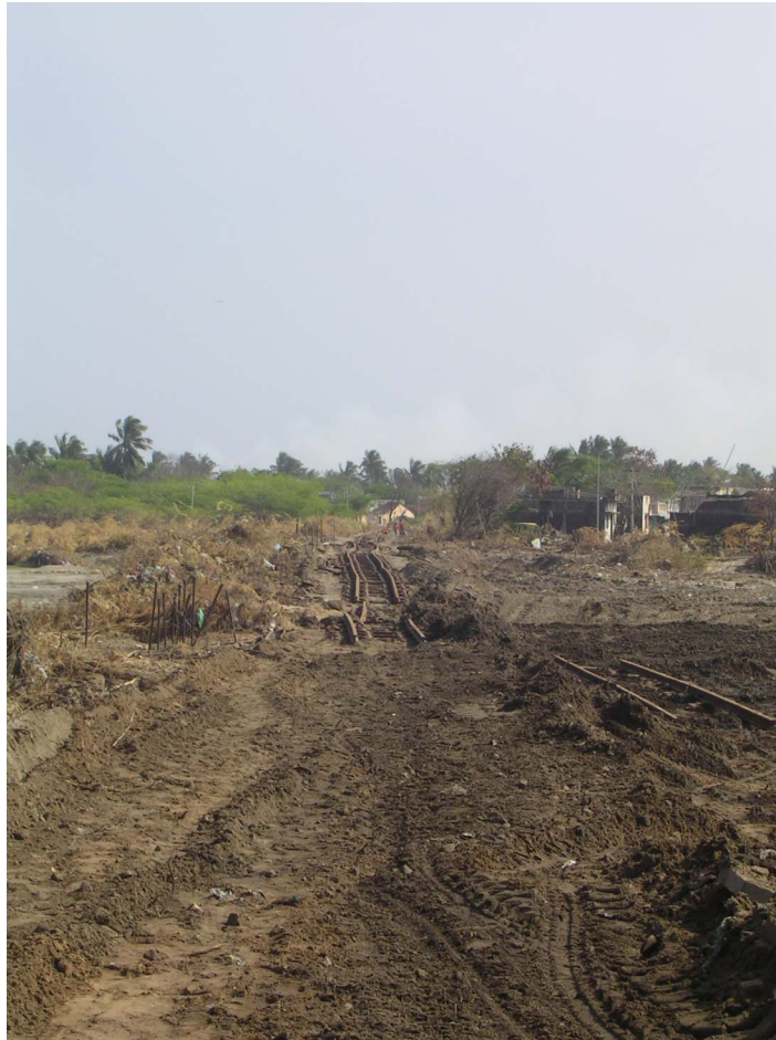
Figure 21. Damaged railway line between Nagore and Nagapattinam (photo: A. Sheth).
