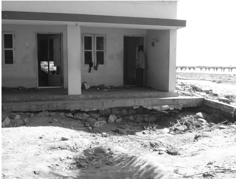
Figure 12. The runup height at Kolachel Beach was 2.6 m, as shown by the watermarks (photo: A. Sheth).
