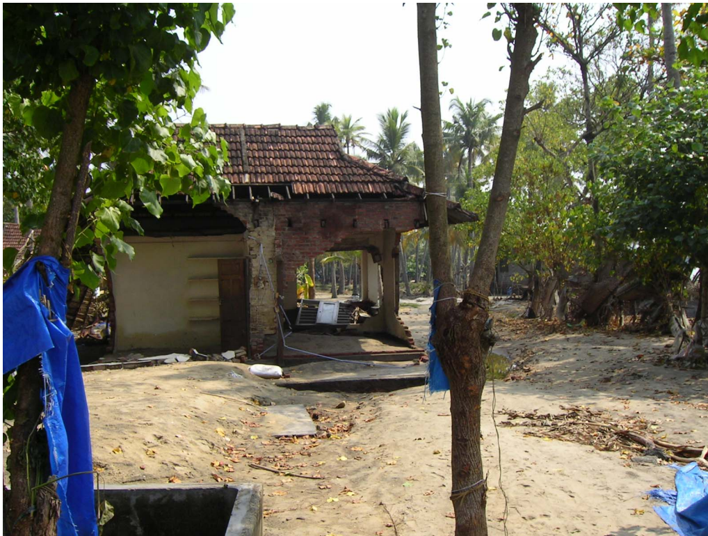
Figure 8. Damaged house in Edavanakkad (photo: A. Sheth).
