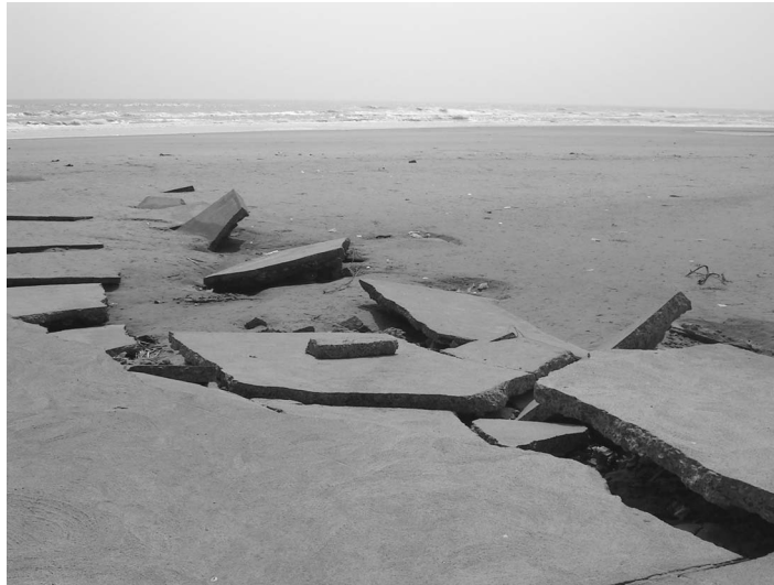
Figure 22. Tsunami waves washed away the newly built roads at Silver Beach, Cuddalore (photo: A. Sheth).
