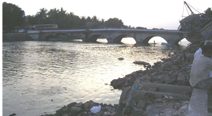
Figure 27. Arasalar Bridge—the two southern arches of this bridge collapsed in the tsunami, but a temporary Bailey bridge was erected by the Indian army within six hours (photo: A. Sheth).
