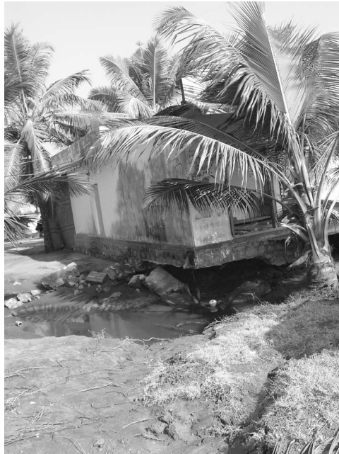
Figure 9. Scouring in Allapuzha—houses were 4–15 m from the shoreline (photo: A. Sheth).
