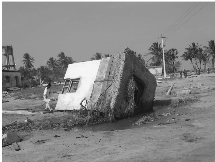
Figure 20. Toppled control room on Ariyanattu Street (photo: A. Sheth).
