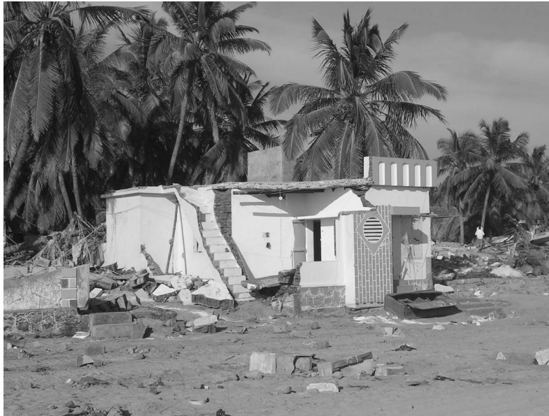
Figure 32. The lack of structural integrity caused failures to trigger at the corners of structures (photo: A. Sheth).
