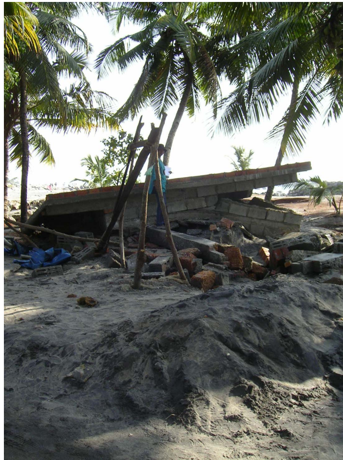
Figure 10. Destruction in the Allapad panchayat —a concrete block house with a reinforced concrete (RC) roof (photo: A. Sheth).
