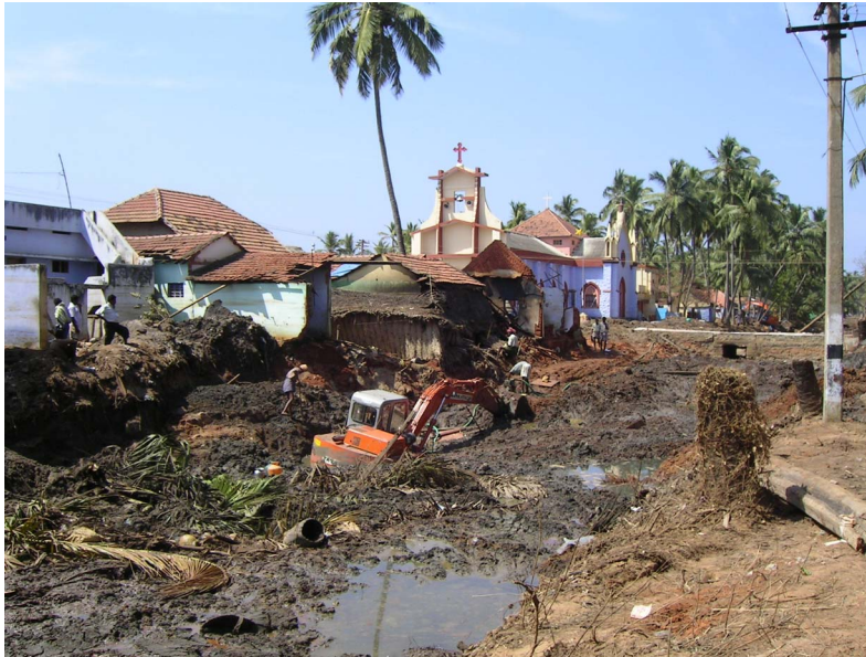
Figure 13. The AVM channel in Kolachel, which became a death trap; more than 300 bodies were found in the slush of the AVM channel and open trenches (photo: A. Sheth).
