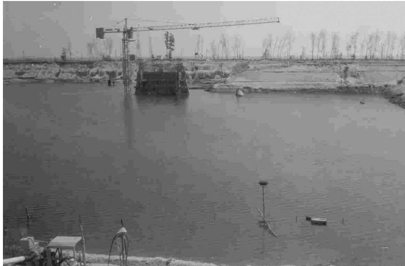
Figure 25. The foundation pit of this 500-MW reactor was inundated by 6 m of water (photo: P. Gandhi).
