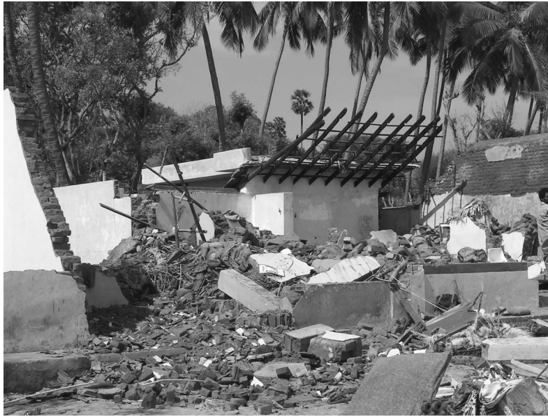
Figure 31. In areas with deeper foundations, masonry superstructures failed first (photo: A. Sheth).
