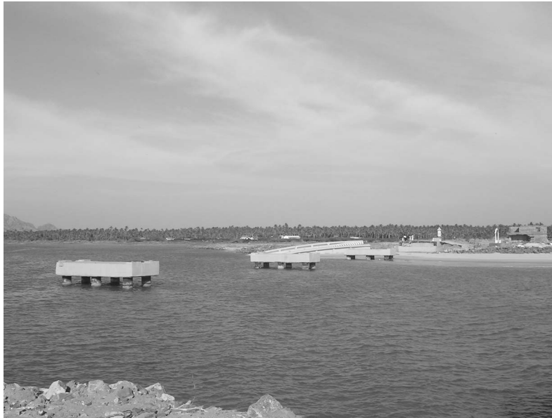
Figure 15. All spans of the Melamanakudi Bridge came off their bearings. The end spans drifted upstream, while the middle spans sank into the river (photo: A. Sheth).
