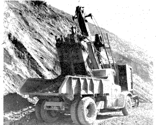
STEAM SHOVEL loads an old seven-yard Bulldog Mack truck at "Old Blue Slide" near Torre Canyon.
