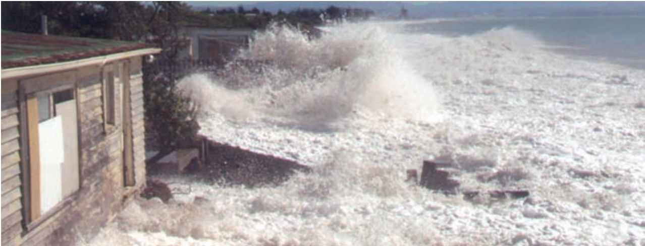
Wave inundation at Haumoana during the Easter Storm (3–4 April 2002). Photo: Hawkes's Bay Regional Council.
