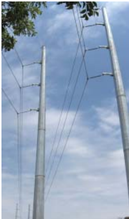
Above and top: Steel towers on the 9-mile Benbrook to Mistletoe route cross everything from a golf course to a railroad yard.
