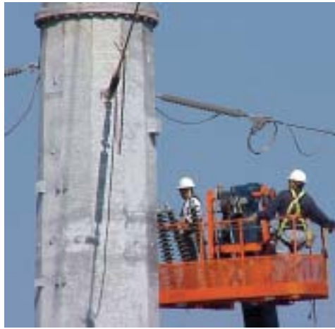
Crews prepare to install insulators on a new steel structure on the 9-mile route from Everman to Handley.
