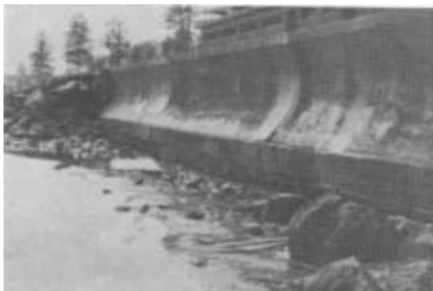
Sea-wall at Broadway, Glenelg After Storm
