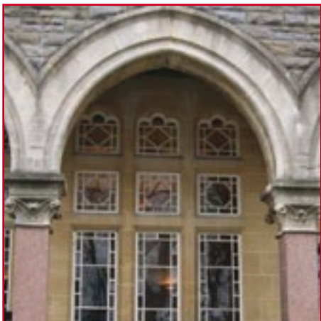
Park House – Pink granite columns and bath stone arches form an arcade on the front elevation.
