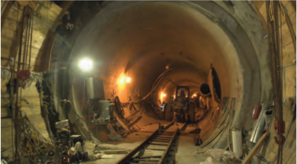
Tunnels that will link the Long Island Rail Road to a Grand Central Terminal station are being dug by two tunnel boring machines.
