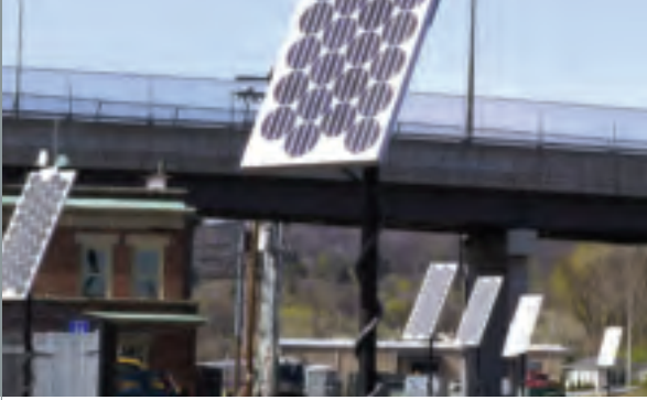
Solar panels at Metro-North's Harmon Shop provide some of the electricity needed to operate the facility.
