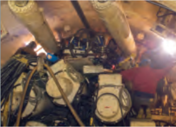
One of the tunnel boring machines at work on the East Side Access project.
