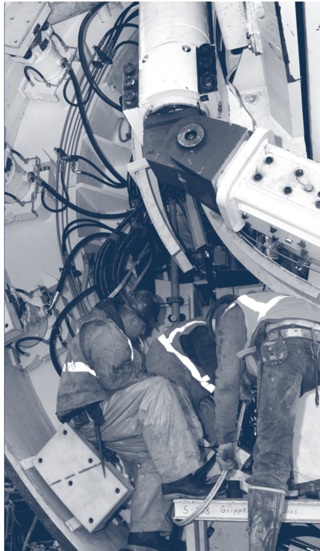
Worker prepares the tunnel boring machine for continued work on East Side Access project.
