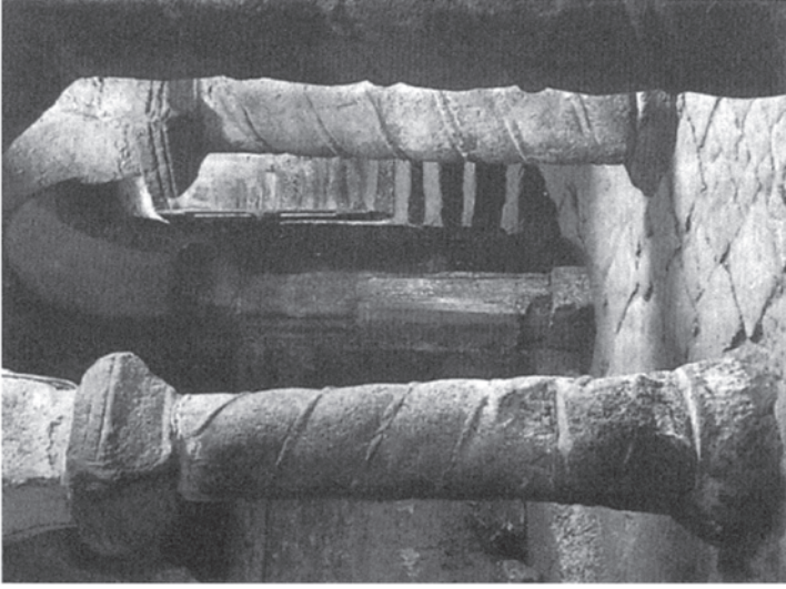
Fig 10. Repton church. The Anglo-Saxon crypt at Repton. (Derbs) showing the pillars which supported the roof and the stairs given access to the several members of the Mercian royal house. The crypt seems to have originated as a freestanding mausoleum, which may have been the burialplace of Æthelbald of Mercia (d. 757), and to have been adapted to form a crypt in the ninth century, perhaps to house the body of prince Wigstan who was murdered in 849 and later venerated as a saint. ( Frank Rogers )
