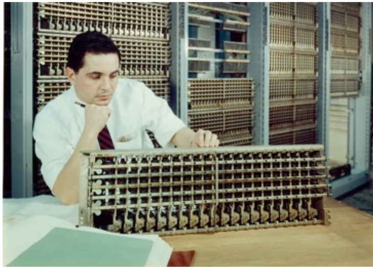
Fig. 5-15. The crossbar switch was developed at Bell Labs and first installed in the Bell System in 1938 and saw service until the early 1990s. The basic switch was a 10-by-20-matrix switch, consisting of electromechanical relay contacts. [1960 photo courtesy of Alcatel-Lucent USA Inc. / Bell Labs.]
