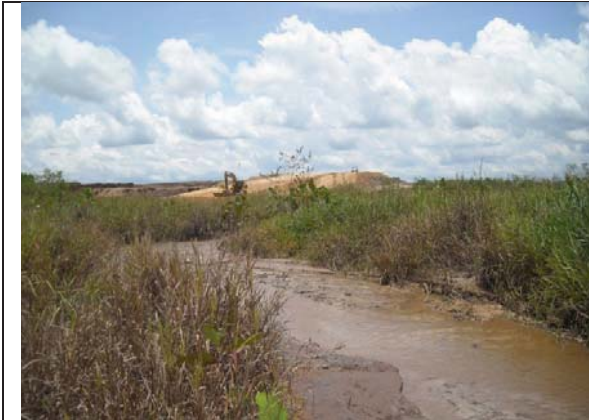
Plate 3.7 Currently on-going site clearing works by other at water sampling location W2.
