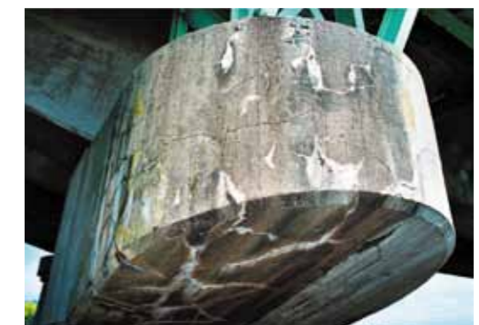
Deterioration due to an alkali aggregate reaction
