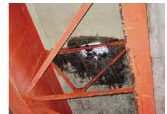
Collapsed slab due to fatigue
