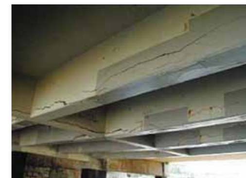
Deterioration due to salt damage
