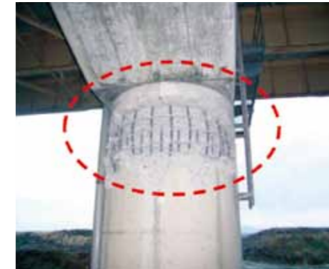
Non-seismically reinforced bridge pier damaged by earthquake
