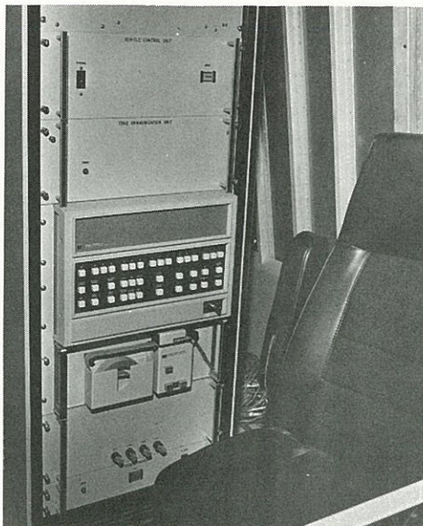
Figure 2-34. Automatic Train Control Equipment Rack
