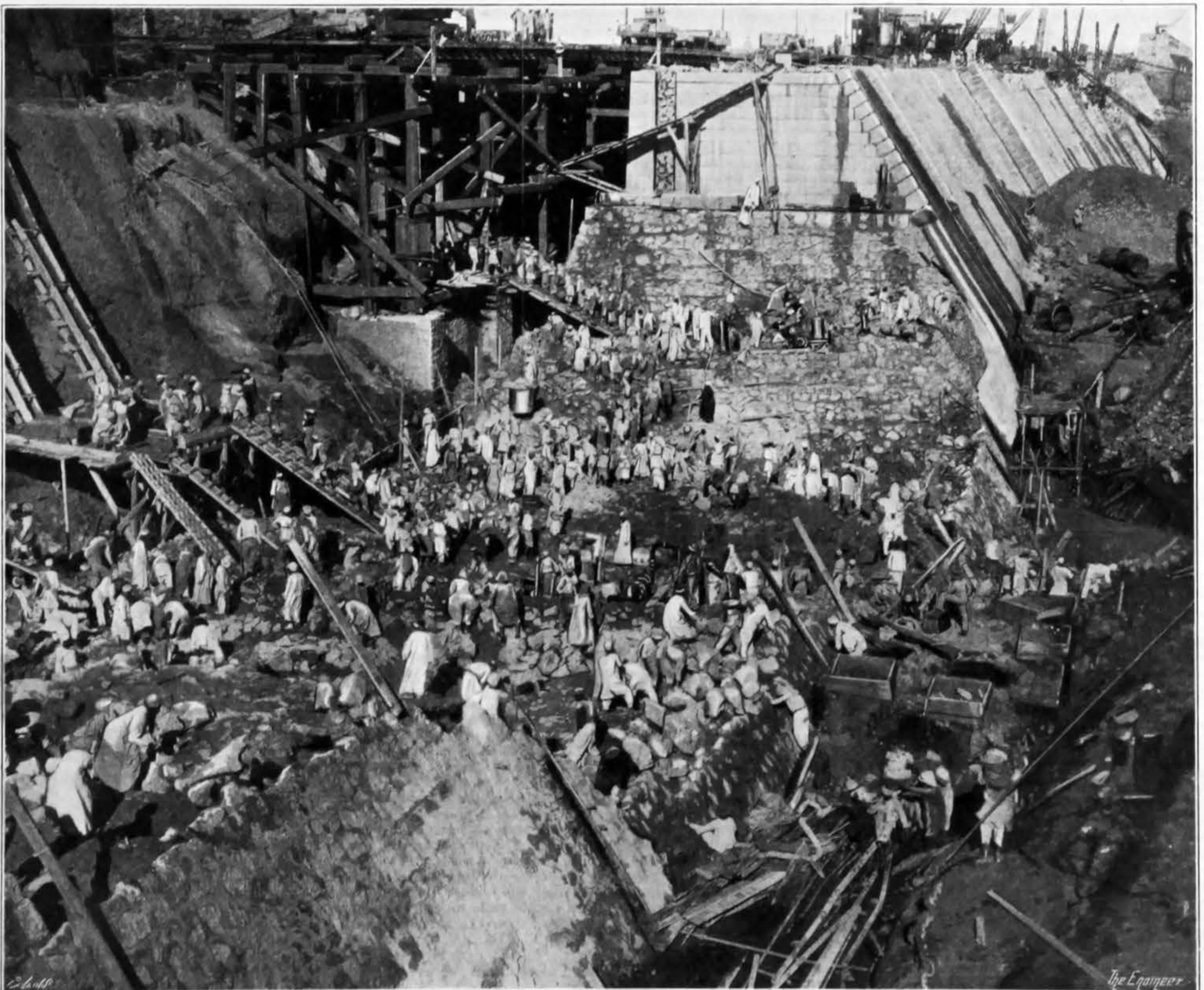
FIG. 5—CONDITION OF MASONRY ABOVE DEEP CHANNEL—JUNE 10, 1924
