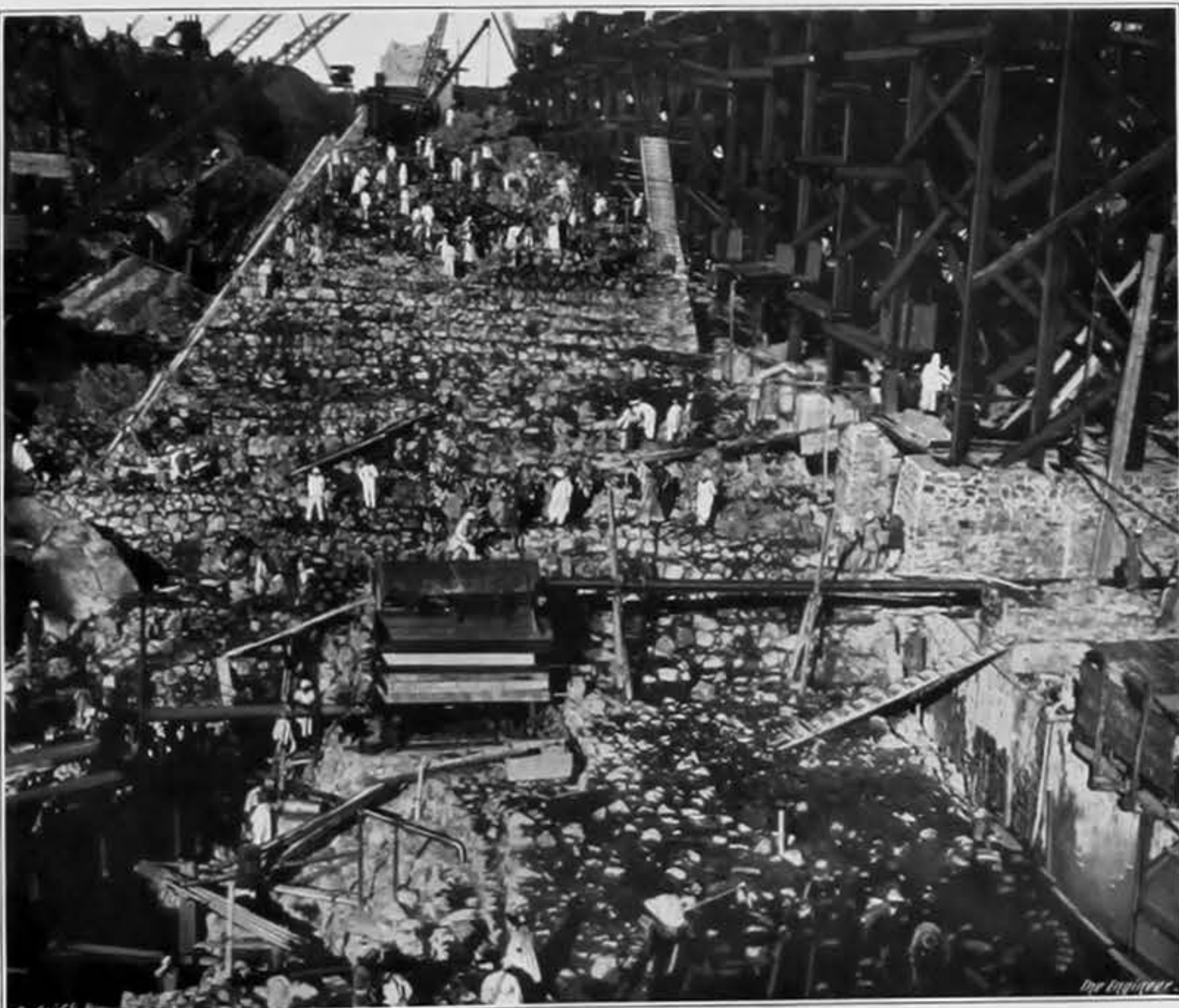
FIG. V.—DEEP CHANNEL NEARLY FILLED IN—MAY 6, 1924
