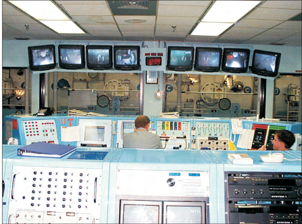
Figure 15-6. NEDU's Ocean Simulation Facility Control Room.
