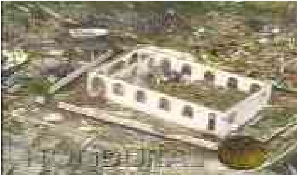
Photo 6. Loss of a roof and damage caused by wind in the Islas de la Bahía.
